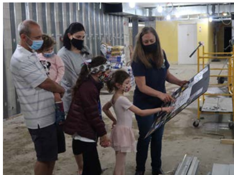
Library Director Kristi Hale shows where windows and french doors will be added to provide natural light and a view to Katharine Wright Park from the new Children's Room.
