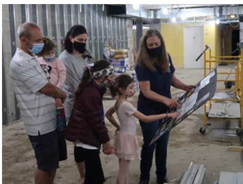
Library Director Kristi Hale shows where windows and french doors will be added to provide natural light and a view to Katharine Wright Park from the new Children's Room.
