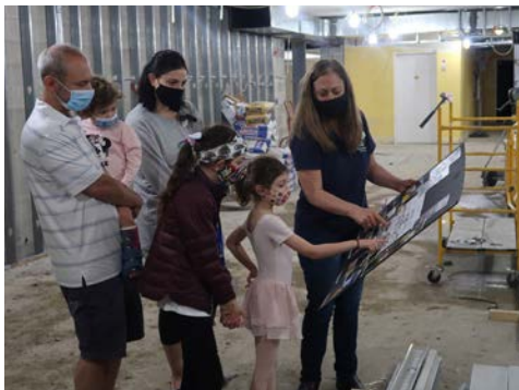
Library Director Kristi Hale shows where windows and french doors will be added to provide natural light and a view to Katharine Wright Park from the new Children's Room.
