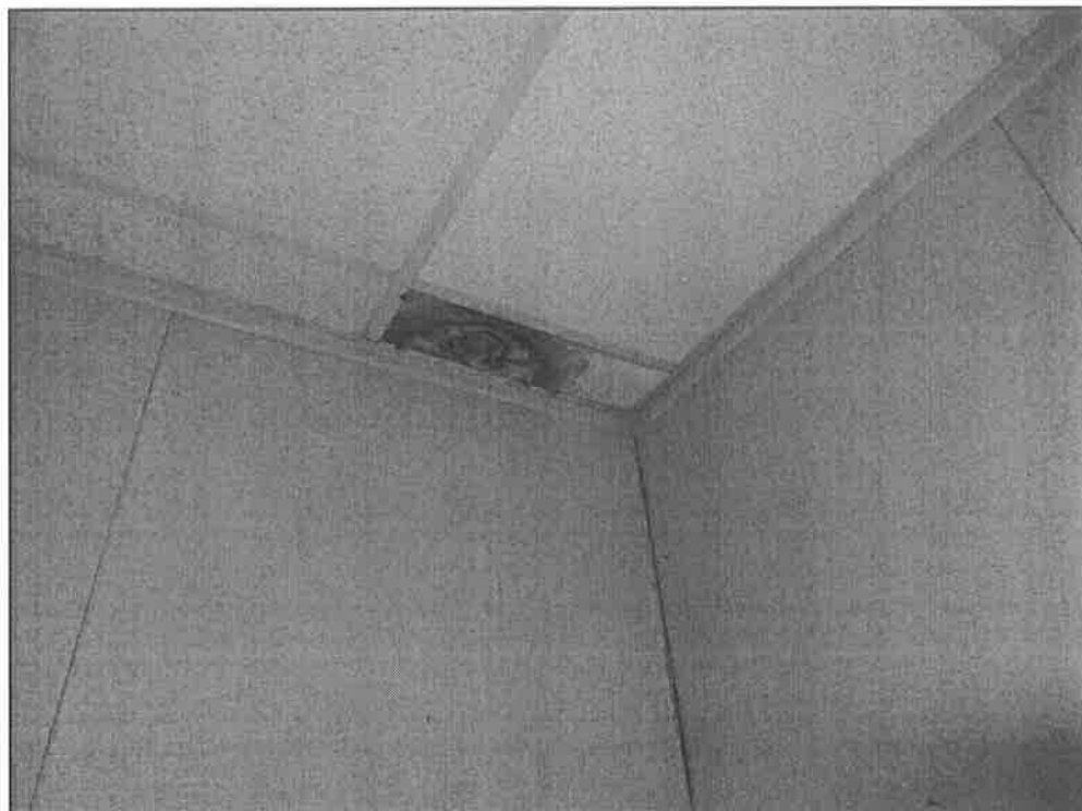
Mold growth in room 107 - location of swab SW-2
