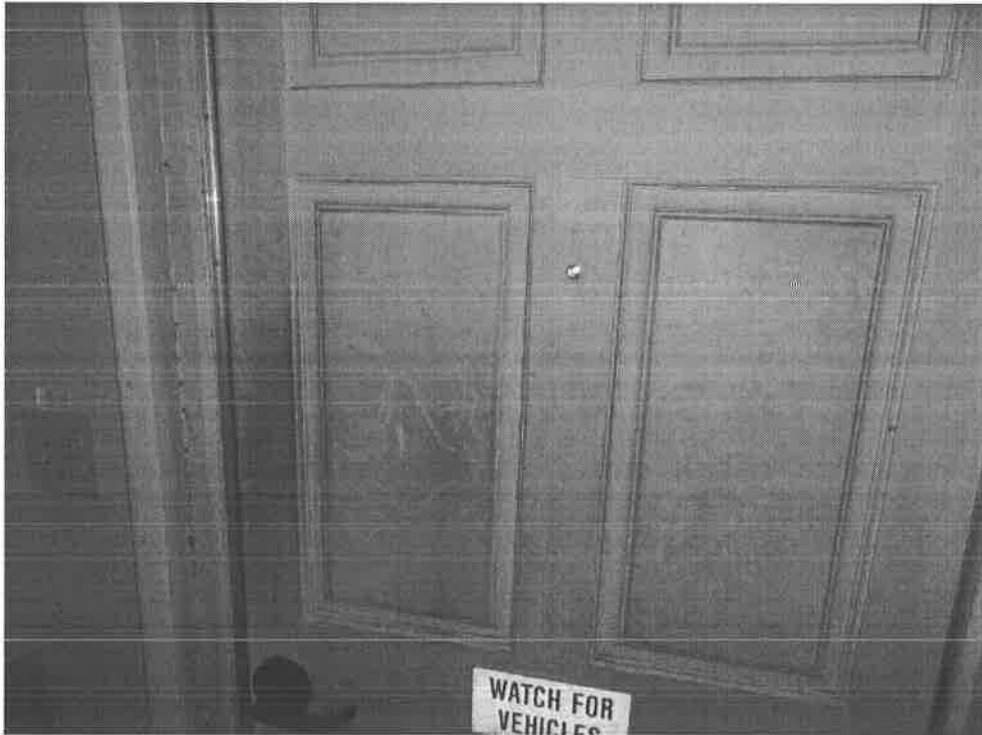
Suspect mold growth on back door
