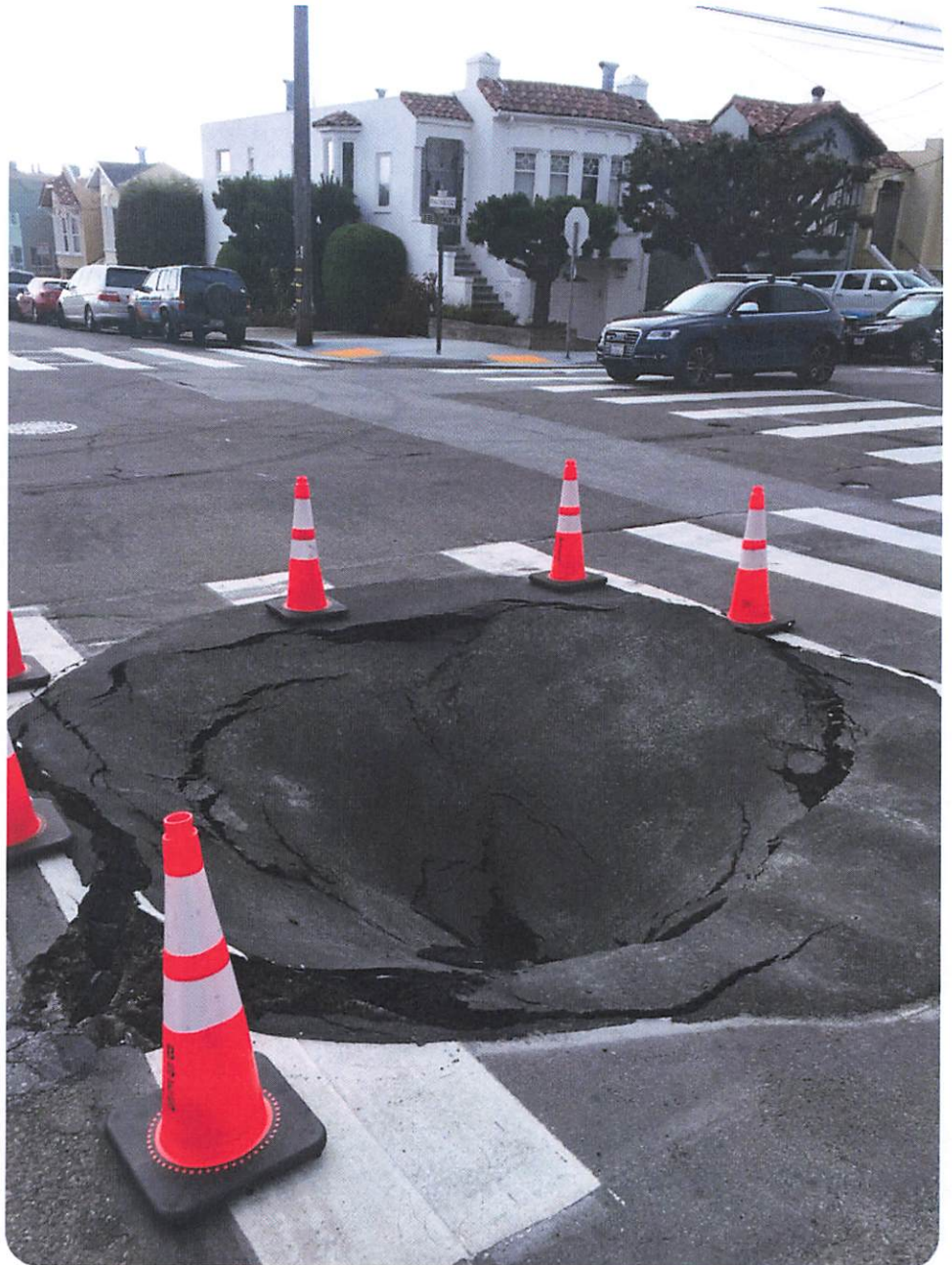
18th and Pacheco Large sink hole, getting deeper.
