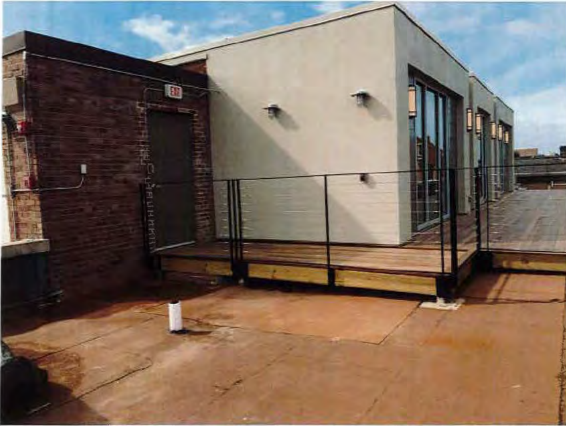
85. Convent roof looking northwest, stair penthouse: in foreground & southeast corner of school at rear
