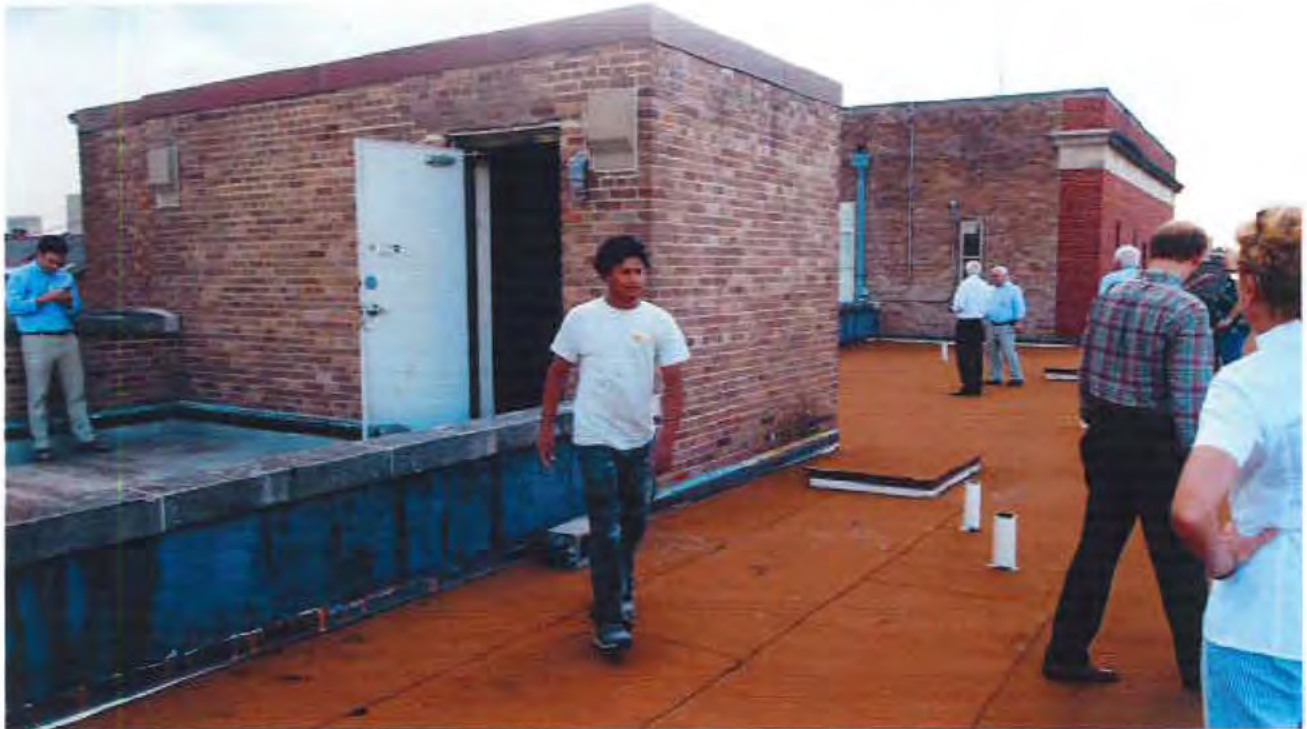
93. Convent roof, looking northwest: stair penthouse in foreground & southeast corner of school at rear
