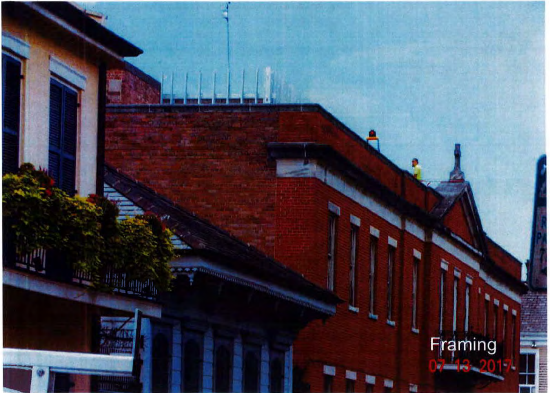
Figure 7: Close-up of the construction photo of rooftop addition from the east on Dumaine Street.
