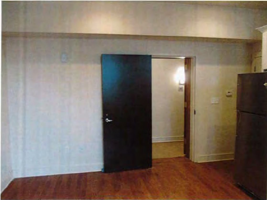
77. Convent. 1 st floor elevator door
